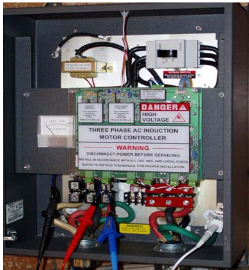
Figure 4. PEC Performance Controller Device
