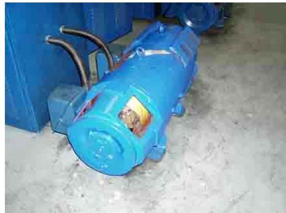
Figure 2. Test Load (Elevator #15 Motor)
